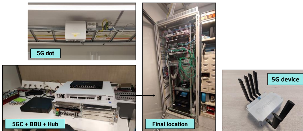
Figure 41. 5G components (5GC, radio, and devices) deployed at ABB lab.
