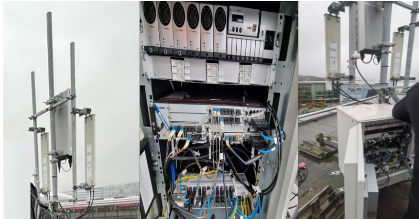
Figure 9: Telenor Research facility radio site at Fornebu.
