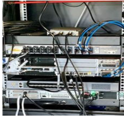
Figure 12: BBU inside the NoW.
