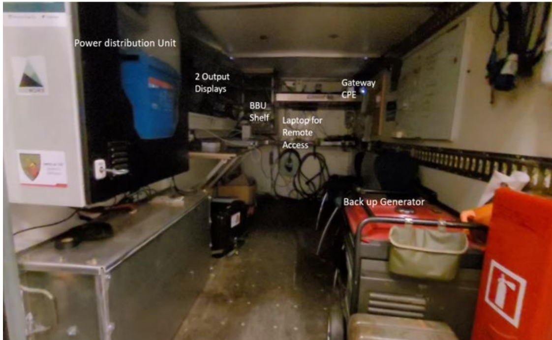
Figure 11: Equipment deployment inside the NoW and AAU shown on the mast outside
