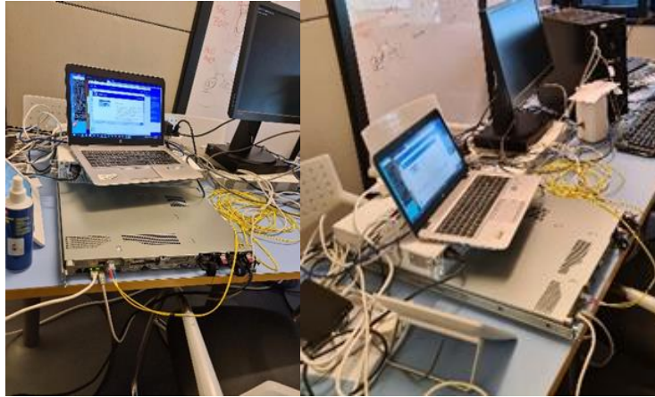
Figure 8: OpenShift deployment in Fornebu Premises.
